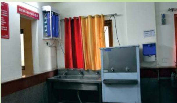
RO Water Facility
