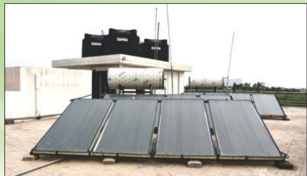
Solar Heating System
