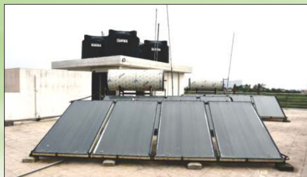
Solar Heating System
