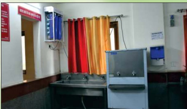
RO Water Facility
